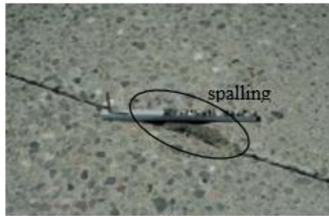
(b) Transverse spalling
