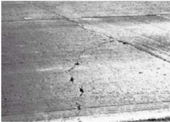
(a) Corner Cracking
