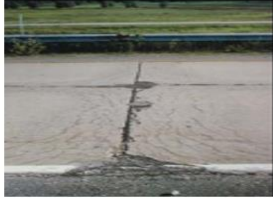
(b) Durability "D" cracking
