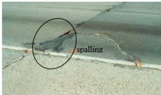
(c) Corner spalling
