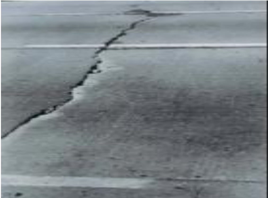
Figure 2.3 Faulting of transverse crack (Source: Miller and Bellinger (2014))
