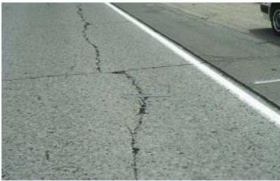
(c) Longitudinal cracking
