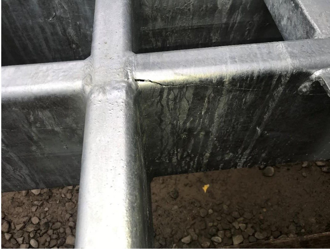
Figure 1.1 An example of material failure during hot-dip galvanizing (Shared with Permission from Sherman + Reilly, Inc.)
